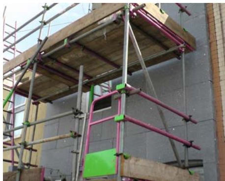
This is decently installed solid wall insulation. But who'd be able to tell if it was a botched job?
