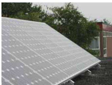
PV array installed with grant from Energy Saving Trust
