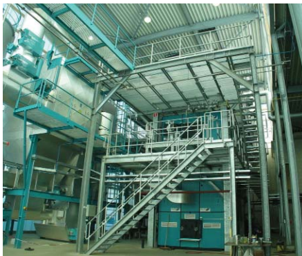
The types of heating systems that Bioheat has in its sights, are large-scale ones such as this.
